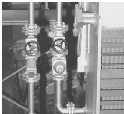
BW installed downstream of an air heater (space heating)
