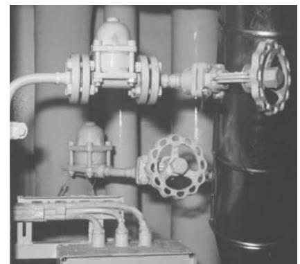
Tank-heating system equipped with BW on an ore carrier
